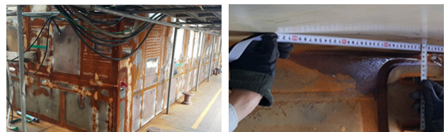
Fig. 1 Failure mode of thin-walled panels in offshore living quarters
