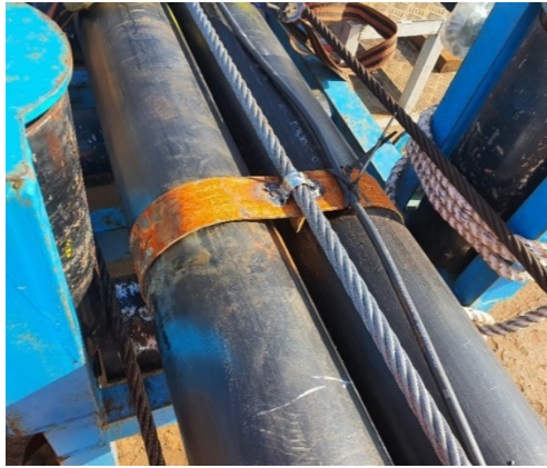
Fig. 10 Water supply pipe
